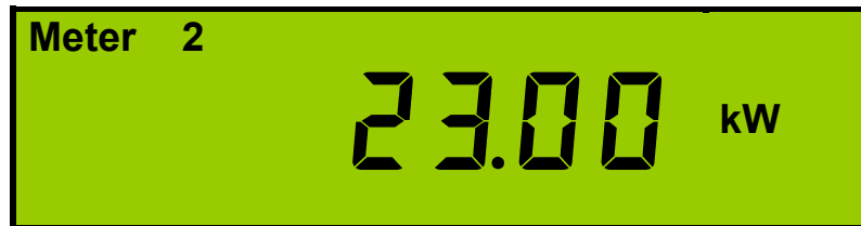
Active Power - Meter 2
